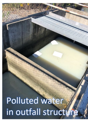
Pumping out illicitly discharged material from outfall
