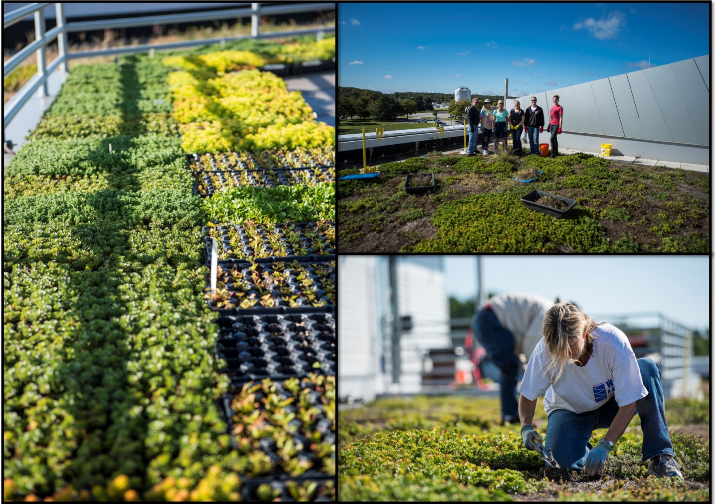
Figure 2 NASA LaRC's green roof on the Headquarters Building (B2101) was restored by volunteers. The roof helps improve water quality and reduce energy consumption.
