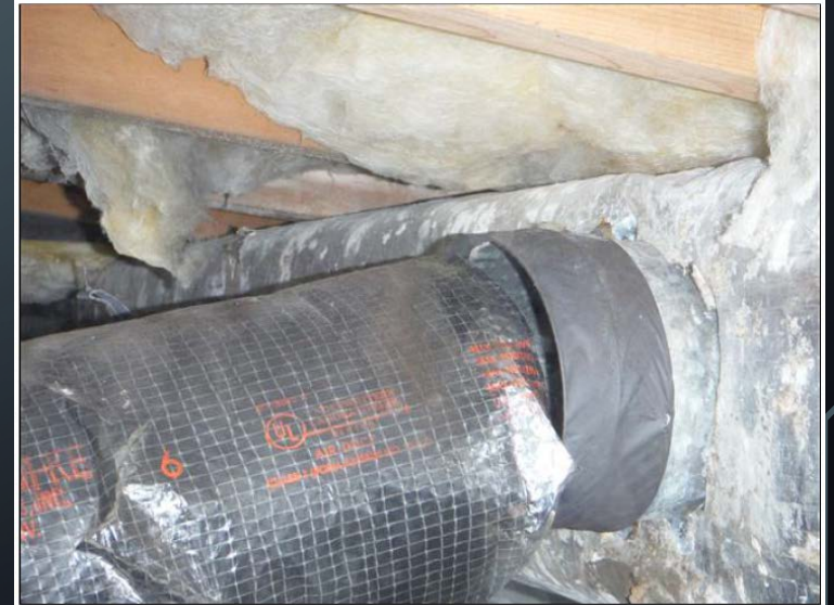
11.4 DUCTWORK Picture 2 Separated Duct Connection at Trunk
