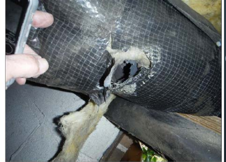
11.4 DUCTWORK Picture 1 Hole in Duct at Crawl Space Door
