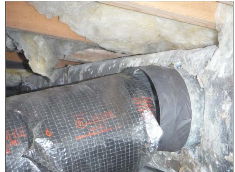
11.4 DUCTWORK Picture 2 Separated Duct Connection at Trunk
