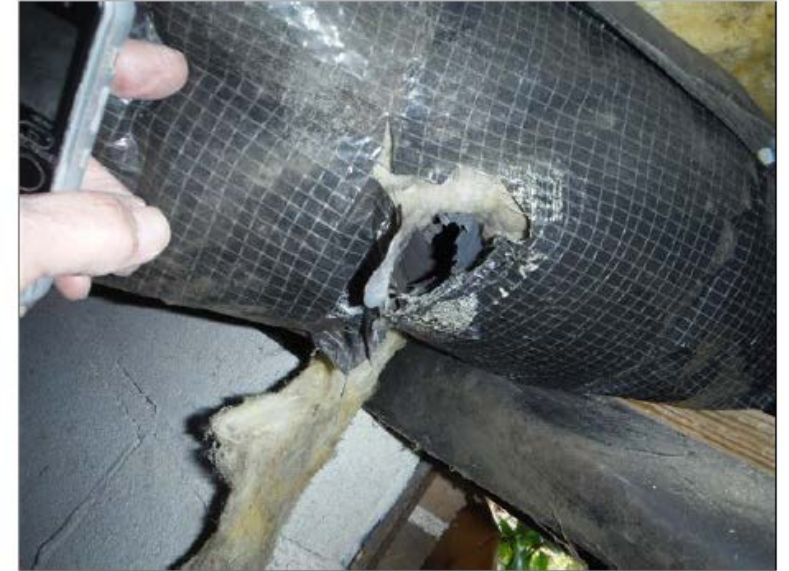
11.4 DUCTWORK Picture 1 Hole in Duct at Crawl Space Door
