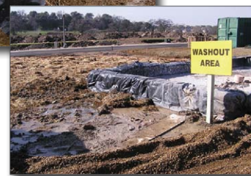
Figure 10. Leaking washout pit that has not been well maintained
